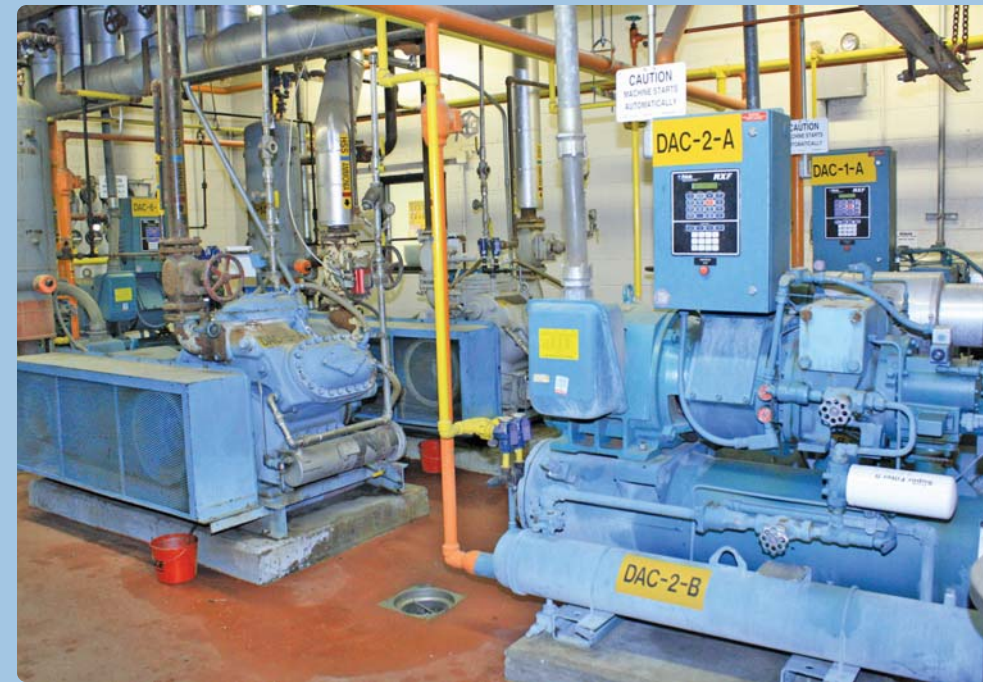
Frick and Mycom Ammonia Compressors
