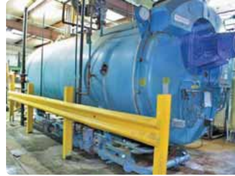
2002 Cleaver Brooks 700 hp Boiler
