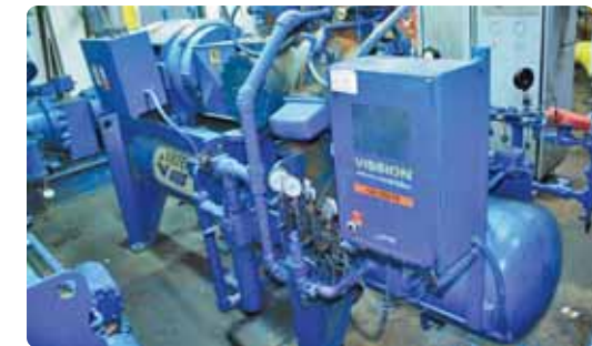
(7) 100 to 600 hp Screw Ammonia Compressors
