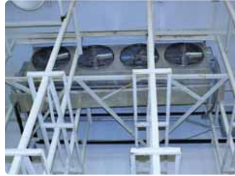
(8) Kramer 4-Fan Freon Freezer Blowers
