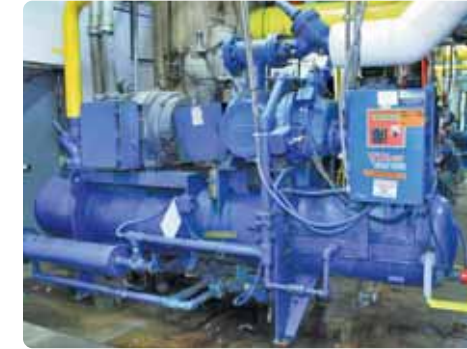
Vilter 400 hp Screw Ammonia Compressor
