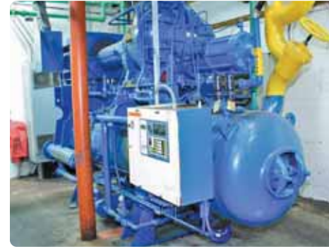
FES 600 hp Screw Ammonia Compressor
