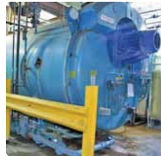
Cleaver Brooks 700 hp Boiler
