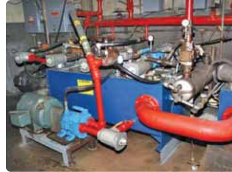
Several Hydraulic Systems
