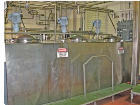
(2) 3 Compartment 500 Gallon S/S Tanks
