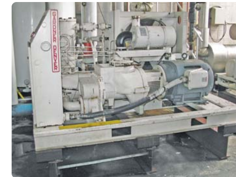
(2) Gardner Denver Air Compressors
