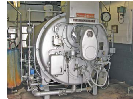
Cleaver Brooks 200 HP Boiler
