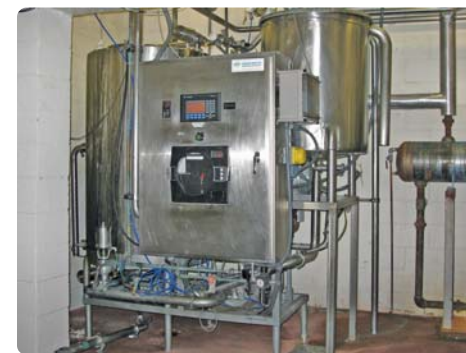
(2) 2-Tank CIP Systems
