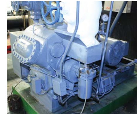
Vilter 8-Cylinder Ammonia Compressor
