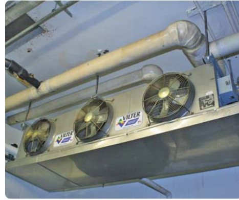
(2) 2008 Vilter 3-Fan Blowers
