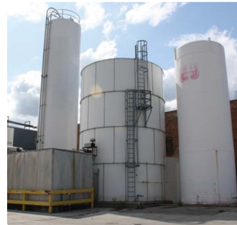
Waste Water Treatment Tanks
