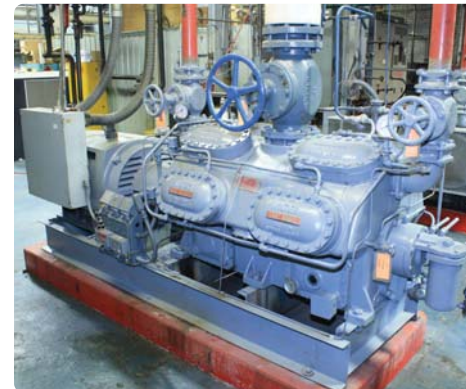
Vilter 16-Cylinder Ammonia Compressor
