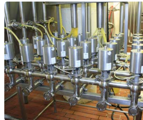
Sudmo 30-Valve Air Valve Cluster
