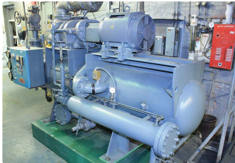
Mycom 100 hp Screw Ammonia Compressor
