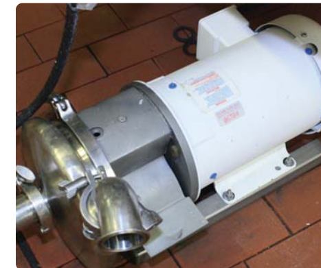
Over (30) Centrifugal Pumps
