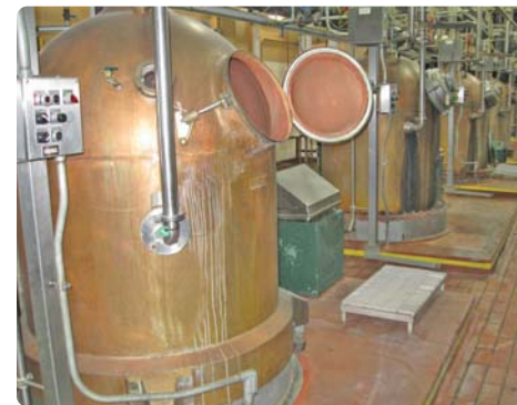
(10) Vendome/Arthur Harris Copper Condensers
